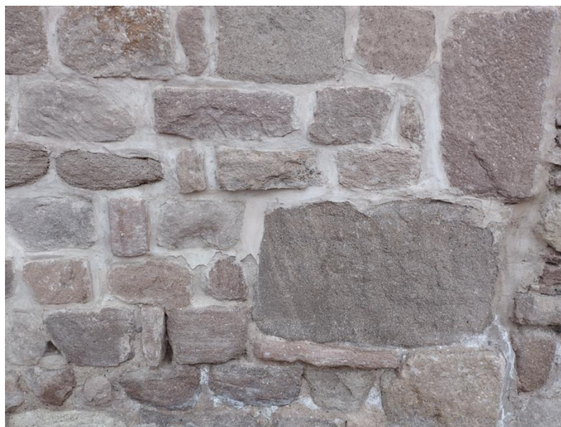
Figure 4. Mortar losses in monument joints
